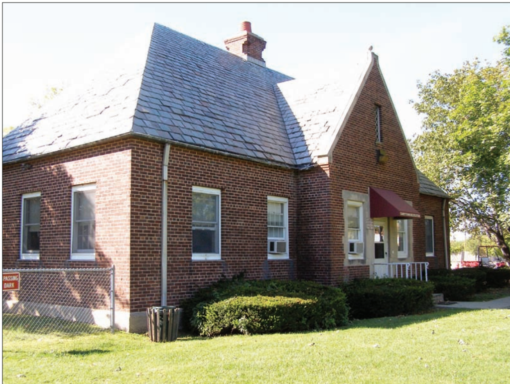
Photo 2. Looking toward east and south façades of the former Administration Building. Note hipped roof with projecting, slate-clad cross-gable, and windows and door in cast stone surrounds.
