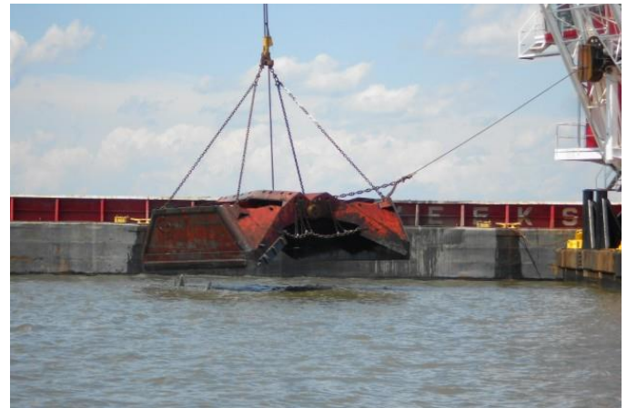
TZC used specially designed clam-shell buckets during dredging operations from August to November.
